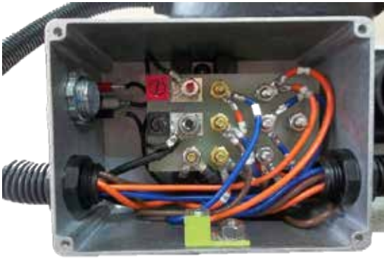
Example of series delta wiring
